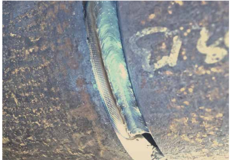
IAC - Vertical downward welding of a root pass in a district heating pipe. Welding speed is significantly increased compared to traditional upward welding..
